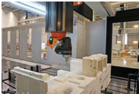
The Zayer TEBAS 6000 5-axis machining centre installed in the new Tryout Center at Audi Tooling Barcelona, Martorell
